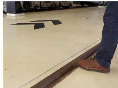
4 RAILS ON THE FLOOR
